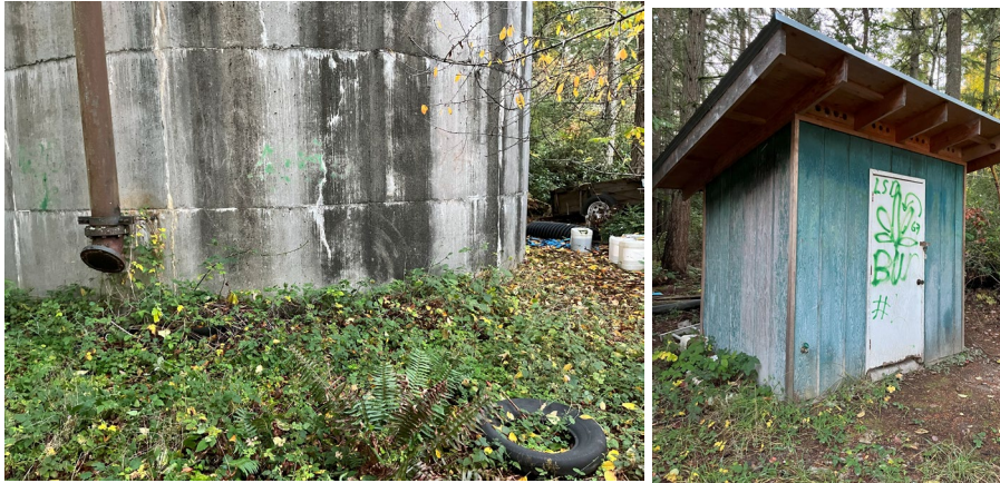
Figure 18. (Left). Tires and debris around tank possibly used to access the tank ladder. Figure 19. (Right) Graffiti on Cove tank PS.
