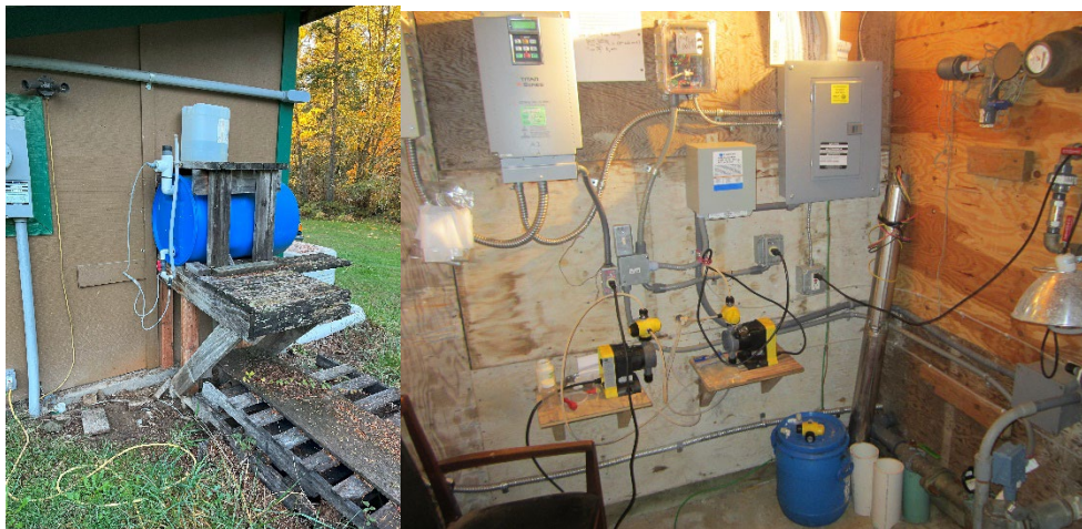
Figure 4. (Left) Hypochlorite Solution set up outside Anderson Wellhouse. Figure 5. (Right) Controls for Anderson Wells.
