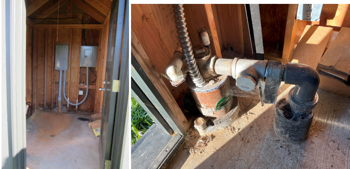
Figure 6. (Left) Well Back40 (S10) pumphouse and controls. Figure 7. (Right) Well Back40 (S10).
