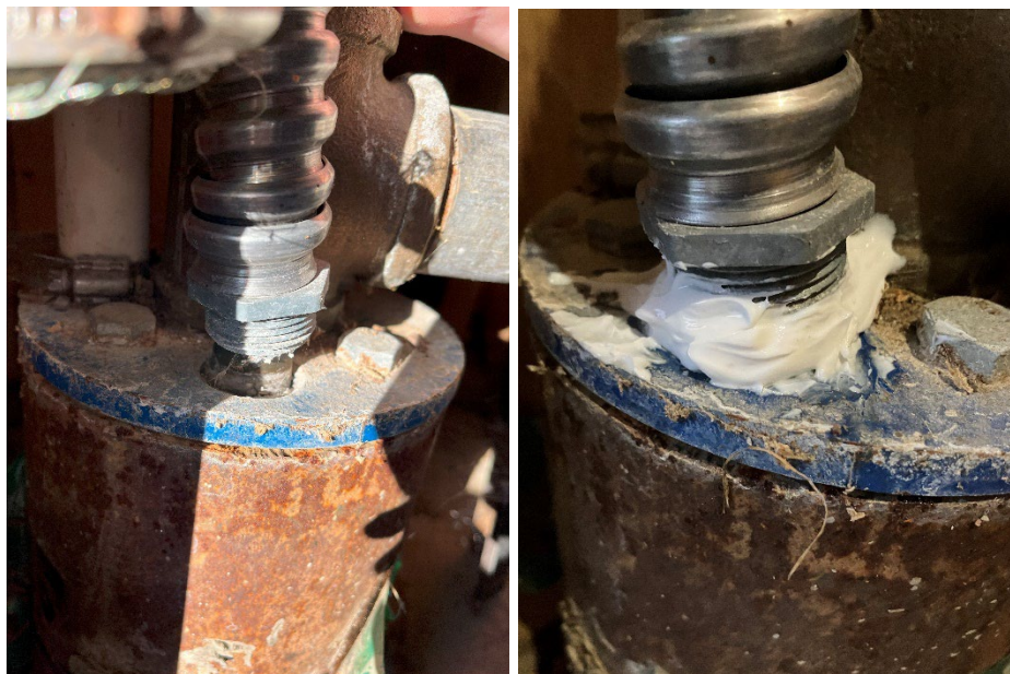
Figure 6. (Left) Loose electrical conduit on Well Back40 (S10). Figure 7. (Right) Sealed electrical conduit on Well Back40 (S10) sent after survey.
