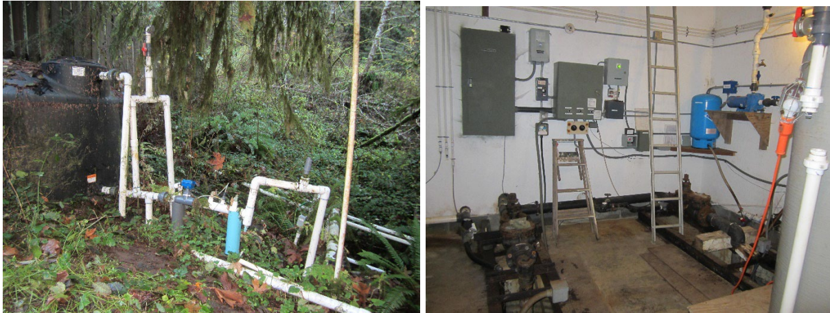
Figure 12. (Left) Springs and wellpoints flow through the 1,100-gallon black collection chamber. Hypochlorite injection is after the overflow and before entering the 15,000-gallon fiberglass holding tank below the Canyon pump house. Figure 13. (Right). Controls inside Canyon pump house.
