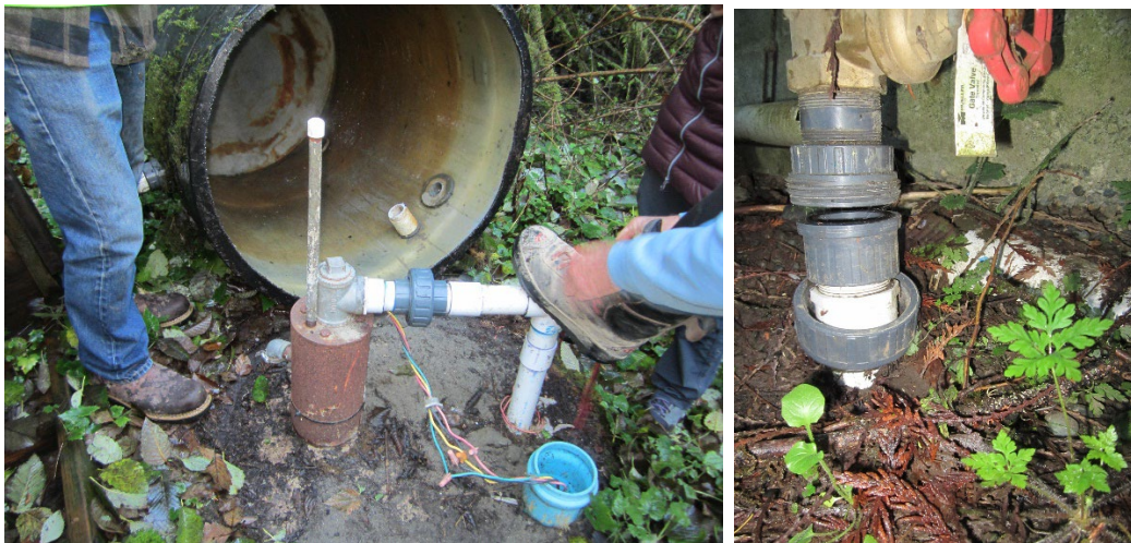
Figure 8. (Left). Canyon Well (S06). Figure 9. (Right). Canyon Well is physically disconnected from the system.
