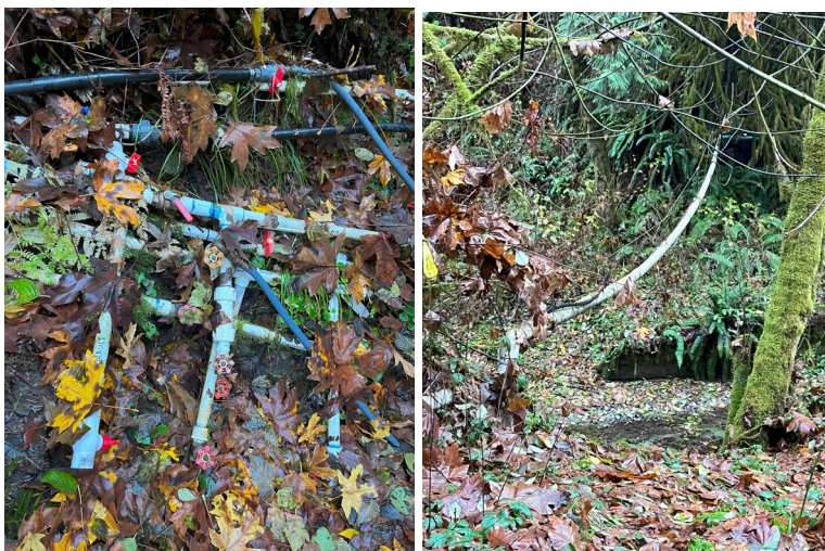
Figure 10. (Left). Wellpoints charging station. Figure 11. (Right) PVC pipe carrying water from springs and wellpoints from across the river.
