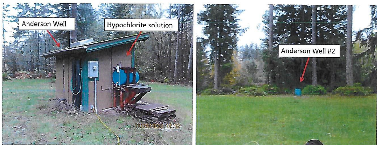
Figure 1. (Left) Anderson Well wellhouse and hypochlorite solution. Think about adding a lock to the door. (Right) View of Anderson Well#2 from the Anderson Well (S07) wellhouse. No potentially hazardous contaminants in the sanitary control area.
