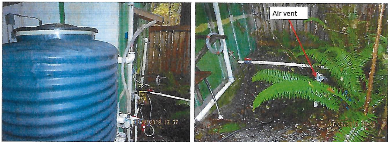
Figure 8. (Left) Blue hypochlorite solution tank. LMI feed pump for the springs and wellpoints on the exterior wall of the Canyon pump house. (Right) Screened air vent for 15,000-gallon holding tank below the Canyon pump house. Treated water is pumped from the holding tank to the Green tank.
