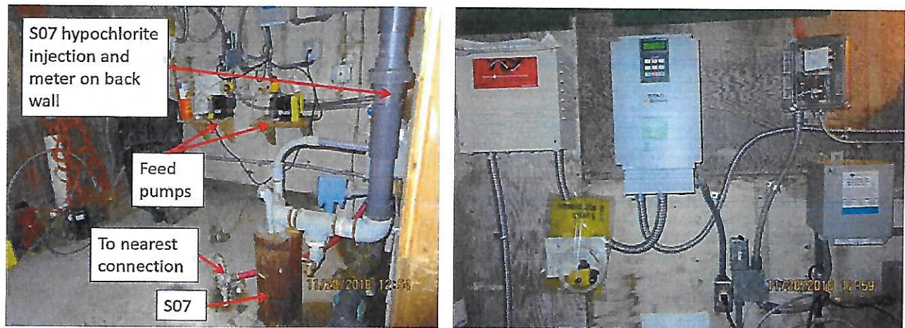
Figure 3. (Left) S07 hypochlorite injection and meter is on the back wall. (Right) Controls for Anderson Wells. Upper right shows the Herrin controller.
