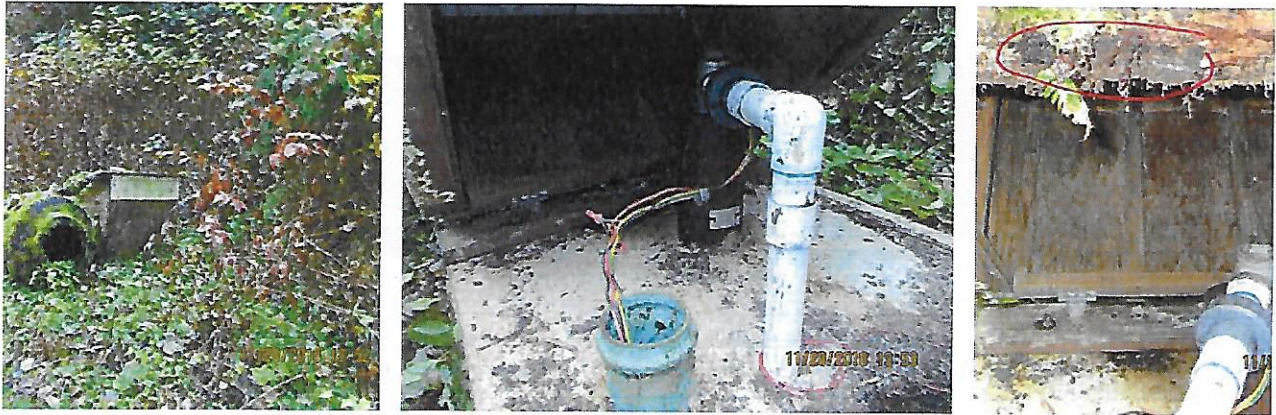
Figure 5. Canyon Well. Source meter and sample tap (not shown here) are located behind the Canyon pump house. (Left) Wellhead enclosure. (Center) Good seals and screens. (Right) Wellhead enclosure front bottom board has rotted and could be replaced.
