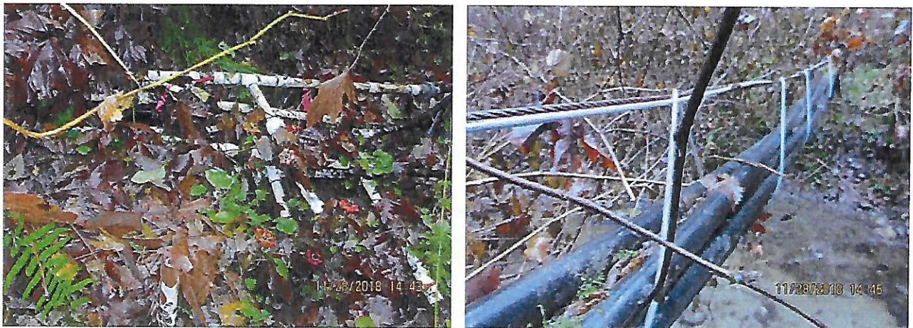
Figure 6. Wellpoints (Left) Charging station. Tap plumbed to the charging station is used to siphon the wellpoint lines as needed. (Right) Wellpoint transmission lines.
