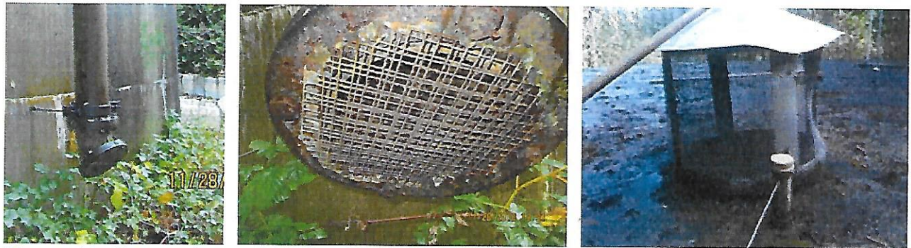
Figure 12. Cove tank. (Left) Overflow airgap. Drain line daylights at roadside. (Center) Overflow screen. Not an adequate insect barrier. (Right) Air vent. Vulnerable to surface splatter and windblown contaminants (photo provided in 2013).
